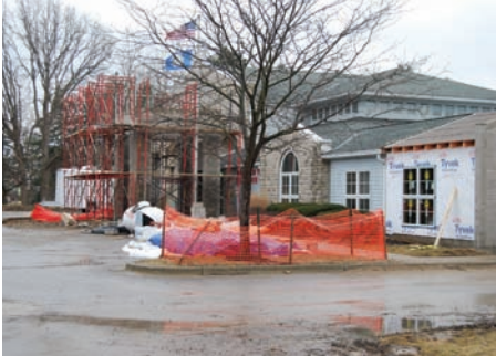
Station 93 at 5825 Brand Road
